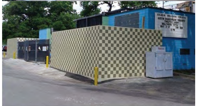
From top: rebar preparation for concrete pour; concrete pour and finishing; project completion - backstage addition; project completion - exterior decorative block walls.
